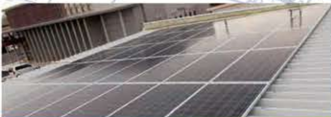
Tokyo, Japan 15kW Rooftop Plant
