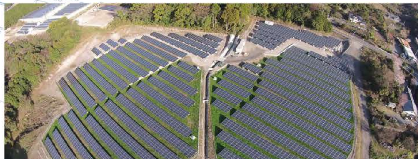
Kumamoto, Japan 1MW Ground Plant
