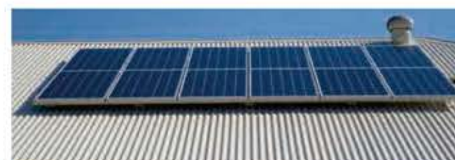
Kelaniya, Sri Lanka 3kW Rooftop Plant
