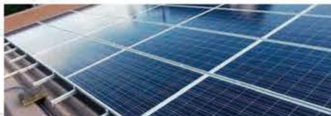
Osaka, Japan 11kW Rooftop Plant
