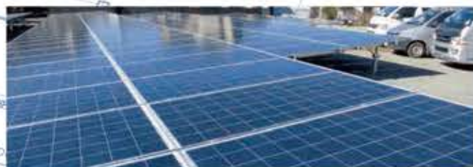
Tokyo, Japan 100kW Ground Plant
