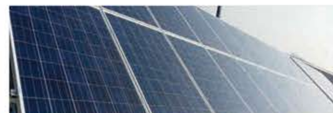
Suzhou, China 200kW Rooftop Plant (Demonstration project)
