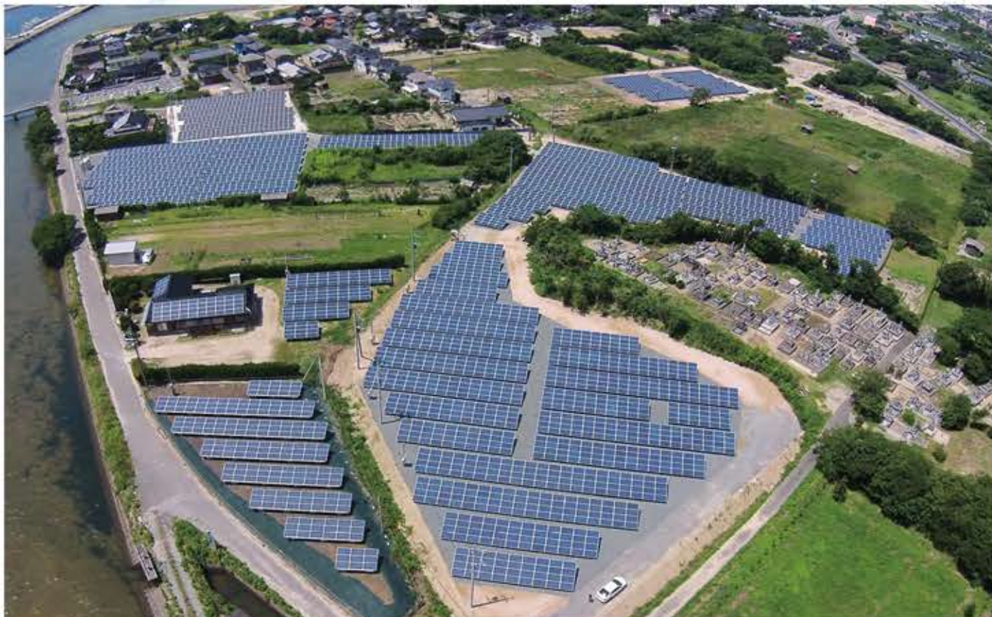
Shimonoseki, Japan 1.5MW Ground Plant
