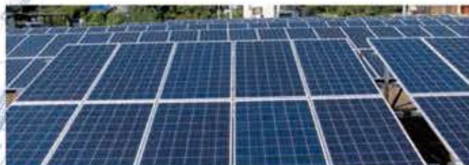
Chiba, Japan 250kW Ground Plant
